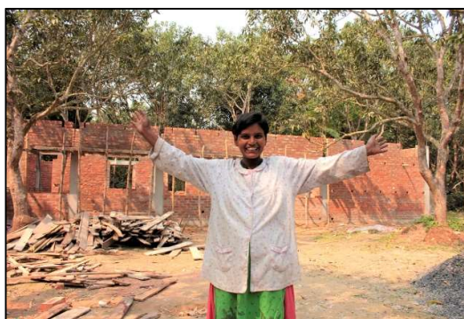
RUPA STANDS IN FRONT OF HER NEW HOUSE UNDER CONSTRUCTION NAYAGRAM IN KASHIPUR IN 2018
